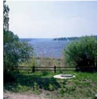
Bank filtration abstraction well, lake Wannsee
