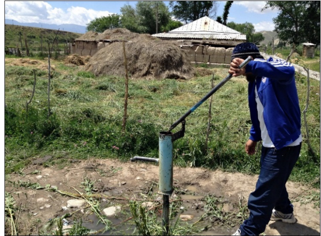
Fig. 2: Hand-operated standpipe in the north-eastern part of Kyzyl-Jyldyz.
